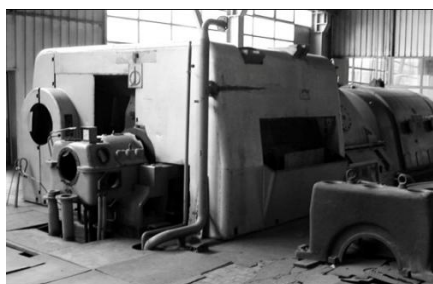
Figure 1. Steam turbine (20 MW) today
