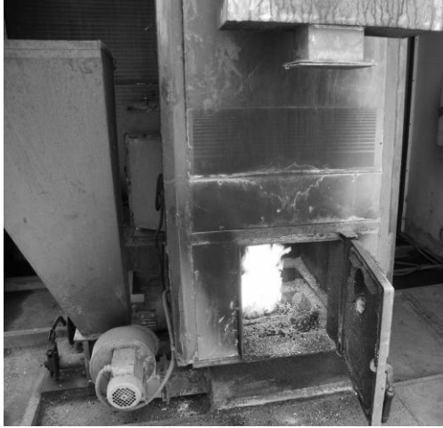
Figure 4. Test of feeding and combustion of crushed maize cobs in coarse wood chips boiler
