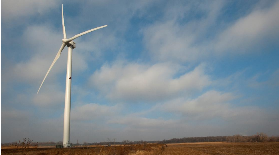
Figure 1. 2.5 MW Clipper Liberty C96 wind turbine, University of Minnesota.
