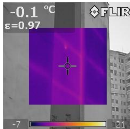
Figure 4. Thermal image of the north oriented façade wall made with FLIR b60
