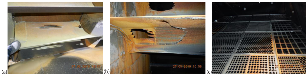
Figure 6. Erosion of the turning vane in the elbow downstream of the horizontal ducts (a), turning vanes in the elbow at the upper end of the vertical ducts (b), and perforated plates in the first distribution grates replaced with plates of inadequate porosity (c)
