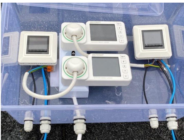
Figure 7. electricity consumption meter and control for model buildings A and B
