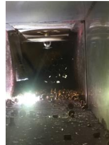
(c) Sprinkler heads with HCP
