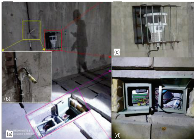
Figure 2. The monitoring system inside the tunnel; (a) the monitoring system inside the tunnel, (b) temperature sensor, (c) the meteorological sensor with five parameters, and (d) data logger [40]
