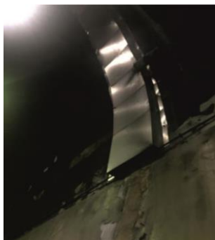
Figure 2. Water box at a leak in the lining
