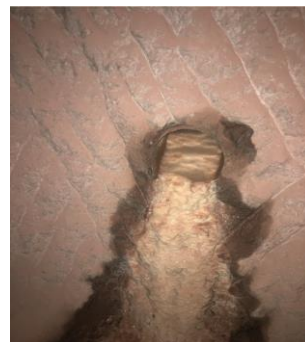
Figure 3. Crystal blockage of a drainage pipe
