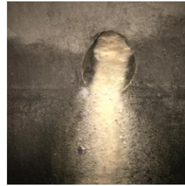
Figure 2. Crystal blockage of drainage pipe
