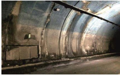
Figure1. Lining cracking and leakage
