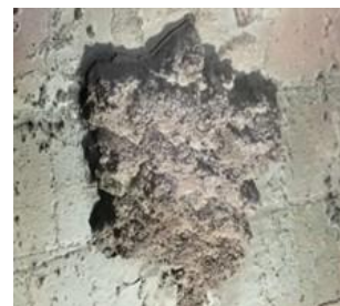
Figure 2 Slags in CFB boiler wall
