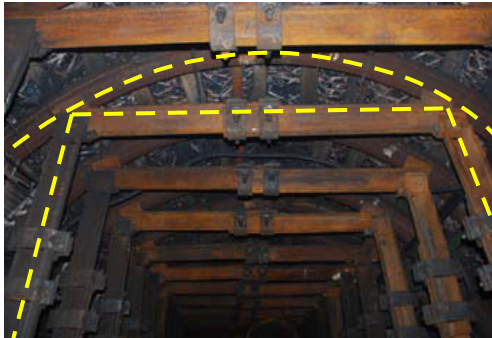
Figure 16. Structurally enhanced U36 steel support
