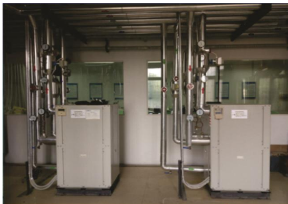
Figure 1. Photo of the GSHP located at Wuhan University of Science and Technology
