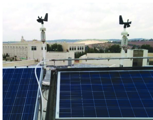
Figure 1. Photograph of PV system and weather station
