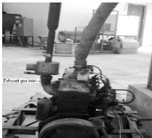
Figure 11. Experimental set-up showing a jet compressor fitted to a diesel engine
