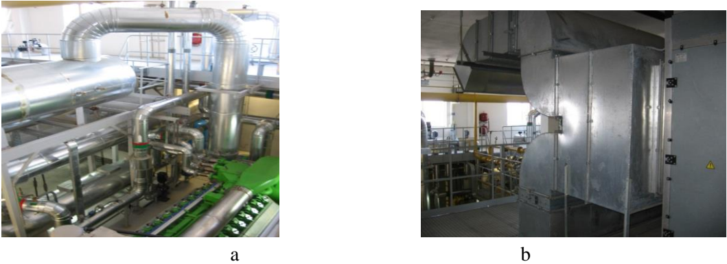
Figure 1. A cogeneration gas engine module (a) and central conditioner for cooling the ambient air, coming into the engine room (b) of IES at the enterprise "Sandora"- "PepsiCo Ukraine"
