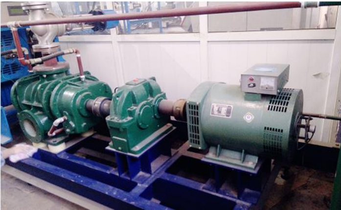
Fig. 11 Test platform of roots type power generation device
