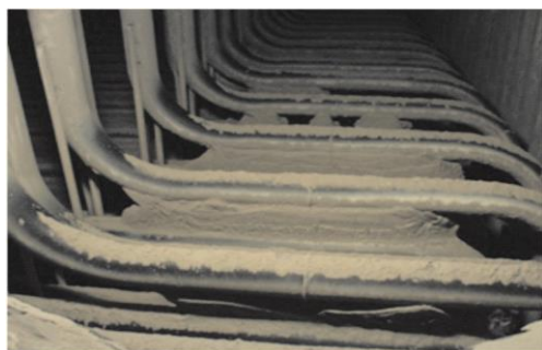
Figure 7. Coils of the first stage re-heater in the second boiler duct fouled by ash
