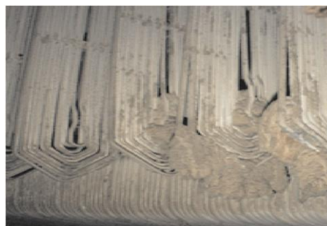
Figure 8. Platen superheater fouled by slag
