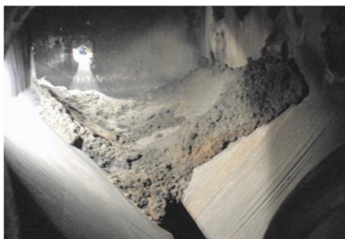
Figure 3. Slagged cold boiler hopper; the slag extends evenly from the bottom of the boiler to the half of height of the burners Nos. 3 and 4 located in the first row
