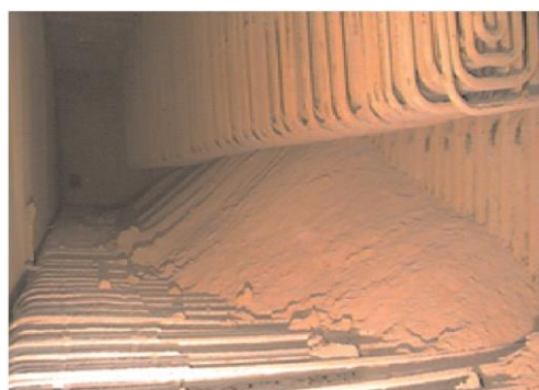
Figure 6. Strongly fouled convective duct (fouled tubes of the IV stage of live steam superheater)
