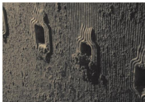
Figure 2. A rear wall of evaporator and OFA nozzles very fouled by slag (level of about 25 meters)
