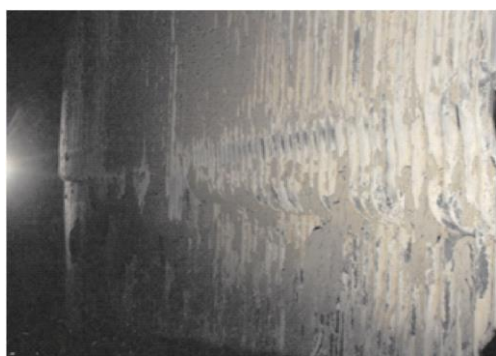
Figure 5. The second stage of the live steam superheater, placed on the front wall of the evaporator fouled by slag
