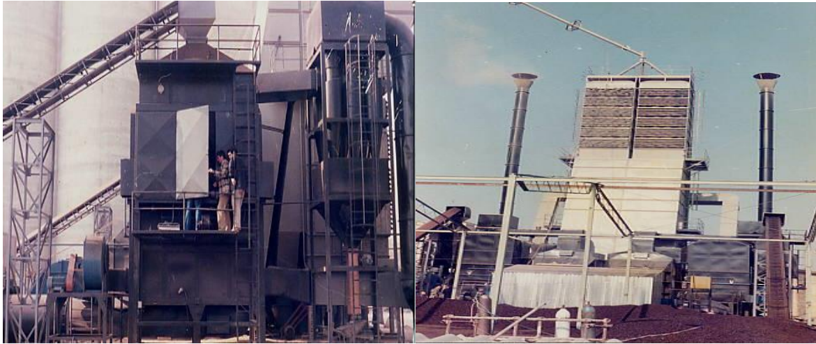
Figure 8. FB furnace (left picture), and the whole facility – twin FB furnaces, vertical corn dryer with coal pile storage in front (right picture).
