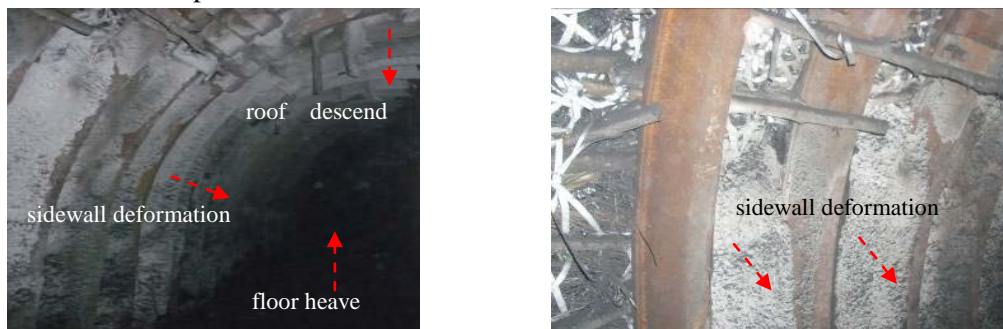
(a) Roadway deformation
