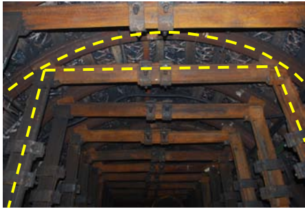
Figure 16. Structurally enhanced U36 steel support
