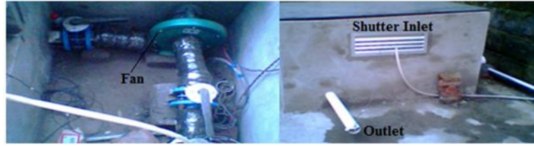
Figure 6. The room for inducing and exhausting air of soil-air heat exchanger
