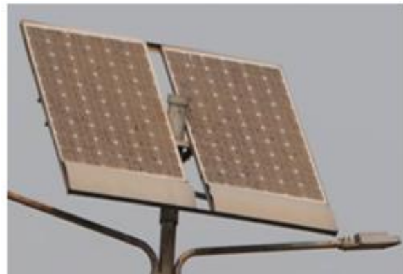
Fig. 2. Pole mounted solar PV installations on GT Road, Mureedkay, Pakistan
