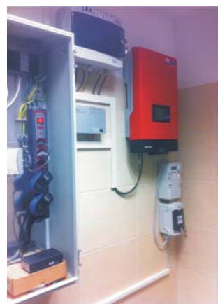
Figure 2. Inverter and the ancillary equipment for the monitoring and data acquisition of PV solar plant
