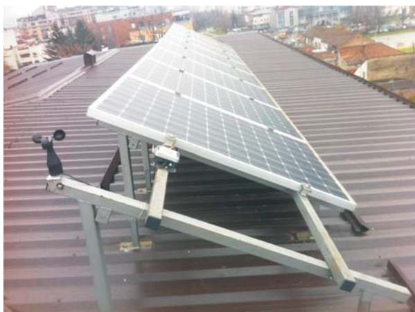
Figure 1. Grid-connected PV solar plant
